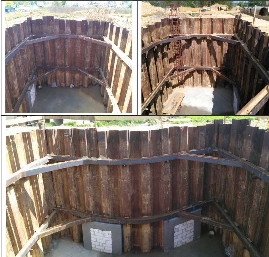
Fig. 1. Technological chamber no.1
