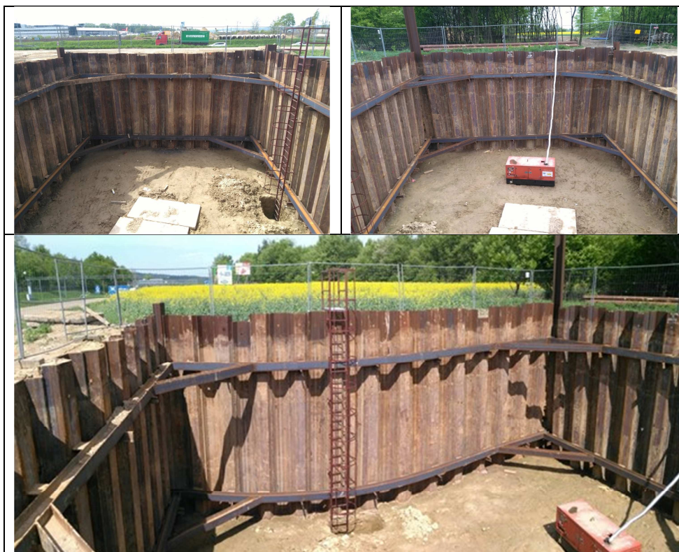
Fig. 2. Technological chamber no.2
