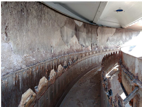
Fig. 4. Corrosion of the concrete wall (left) and the drainage flume overflow ridge steel
