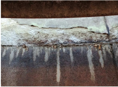
Fig. 2. Destroyed protective coating from the wastewater line upwards
